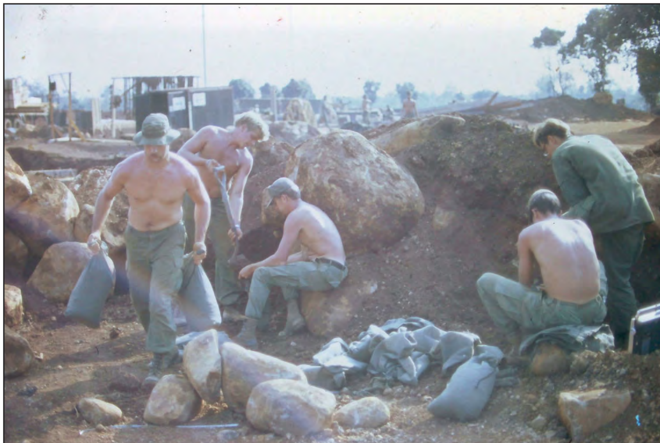
Filling sandbags to strengthen tops and sides of bunkers. This work was never completed. There were always more filled sandbags needed.
