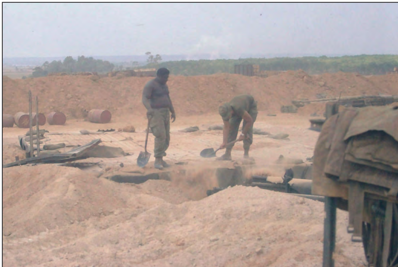
Covering up a row of buried shipping containers to be used as sleeping quarters.
