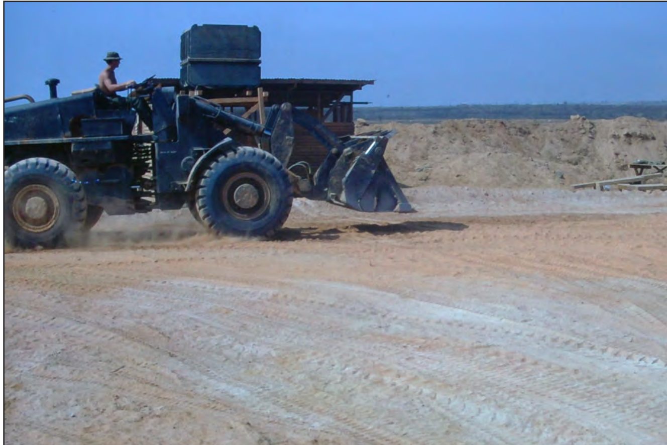
A large front-loader used to scoop up dirt from one place on the base and move it to another place.
