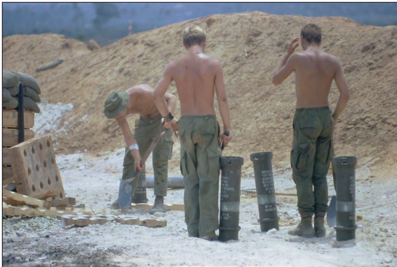
Spreading the new gravel in a gun pit. The board on the left with holes is the top of a transport crate of 155mm shells. It was about 4 inches thick and proved quite useful in base carpentry projects. Another photograph of this thick board being used to protect shells during transport is on page 76.
