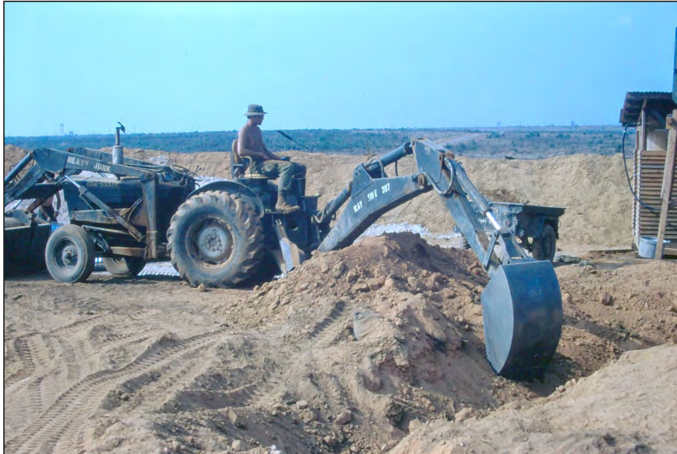
An excavator digger. This particular machine saved us days of time which would have been spend digging drainage ditches by hand.
