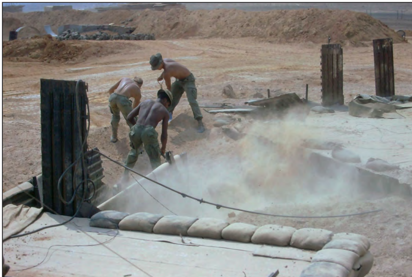
Shoveling dirt to close in the sides of the entrance ramp down into the sleeping area.
