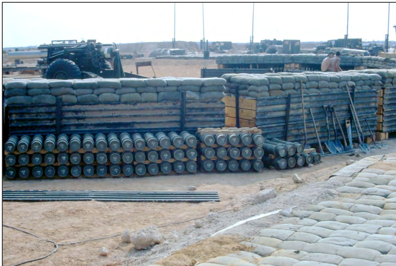
Another view of a rear protective wall of empty powder canisters under construction. Note the row of tools leaning against the rear of the ammunition storage bunker on the right.
