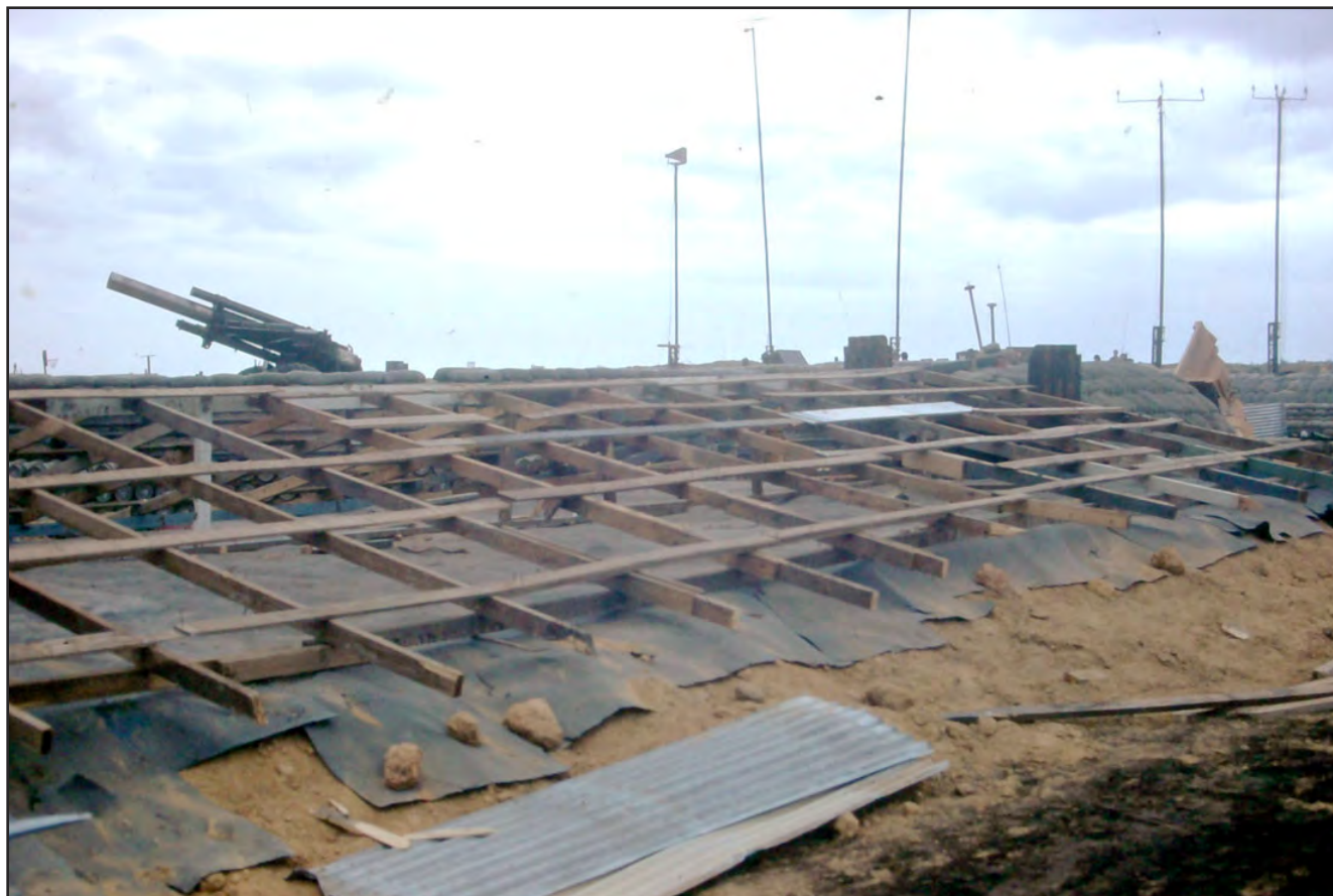
Some sections of the underground sleeping areas were protected from rain water by rolls of tar paper and a roof of light metal sheets. Underneath the tar paper are several layers of sandbags. Note the 155mm howitzer in the left rear of the photograph.
