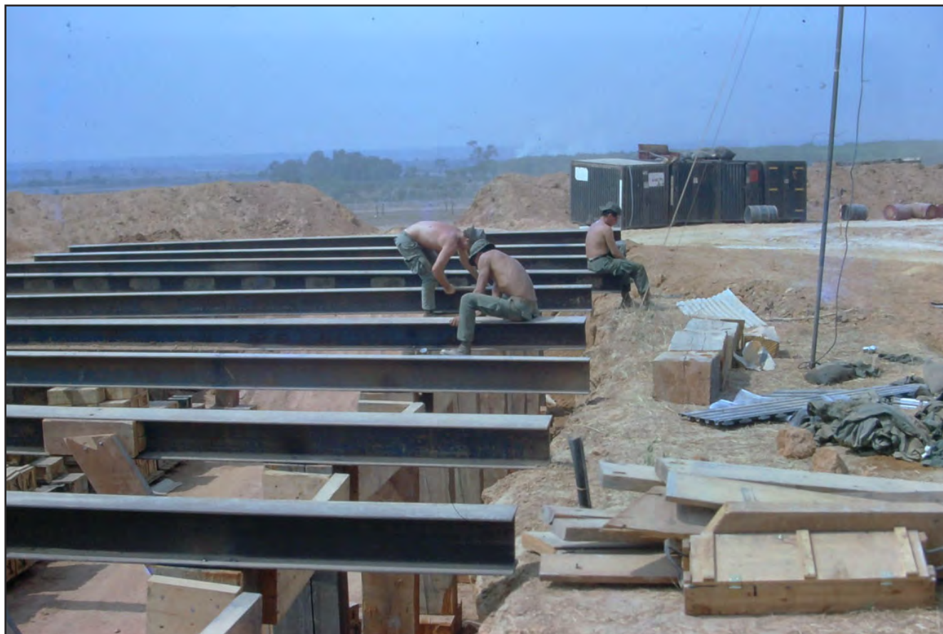
Another major construction project on this fire base was the main ammunition dump. Note the steel girders brought in to form the base of the roof.
