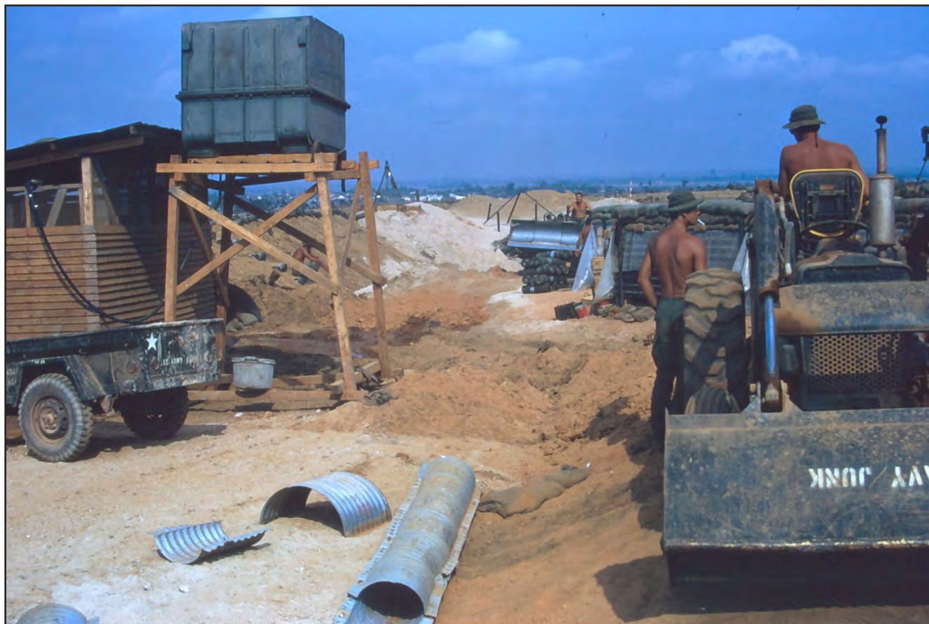
The shower on the left had a large water tank on a tower beside it. More work on the systems of drainage culverts is underway on the right.
